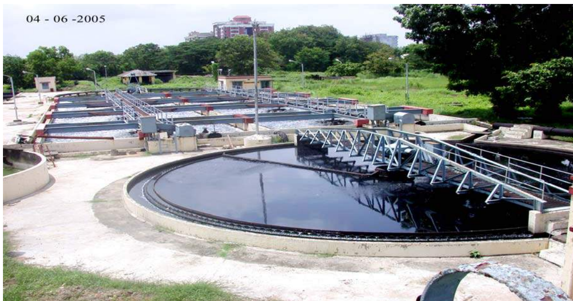
Figure 5.4: 4.50mld Capacity Seweage Treatment Plant (Existing at Elamkulam)
