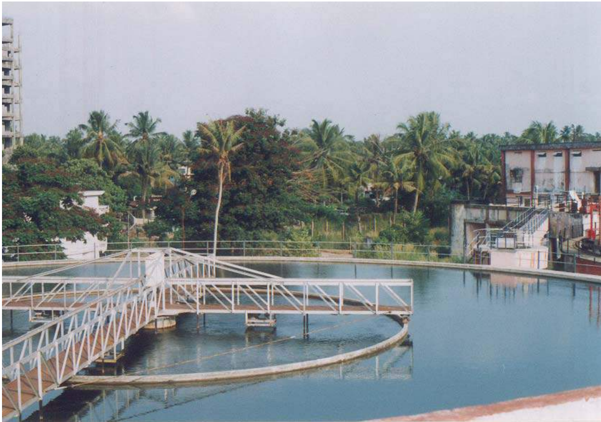
Figure 5.3: Treatment Plant at Aluva
